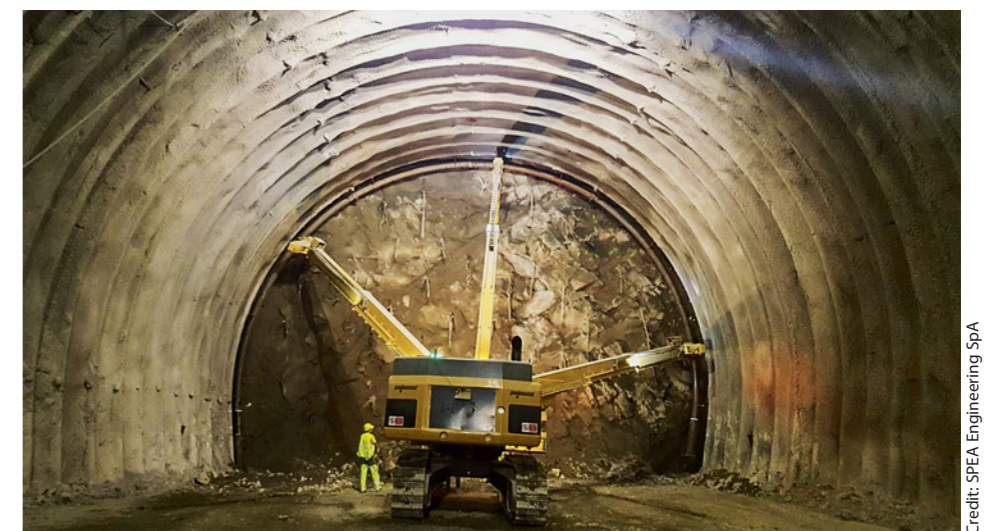
10 Posa centine e adesione centina al profilo di scavo Arch rib placer and adhesion of the arch rib to the tunnel profile
