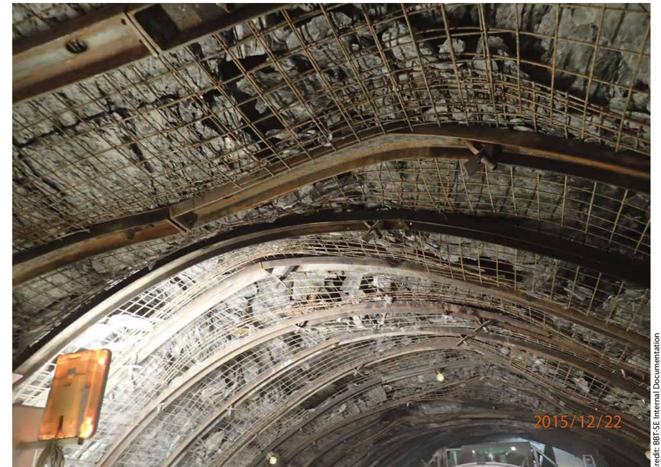
9 Rupture of the support due to overload
