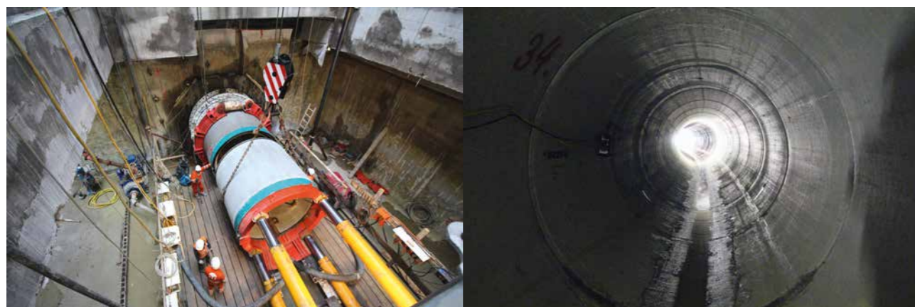
23 [a] The micro TBM and [b] a view of the implemented micro tunnel
