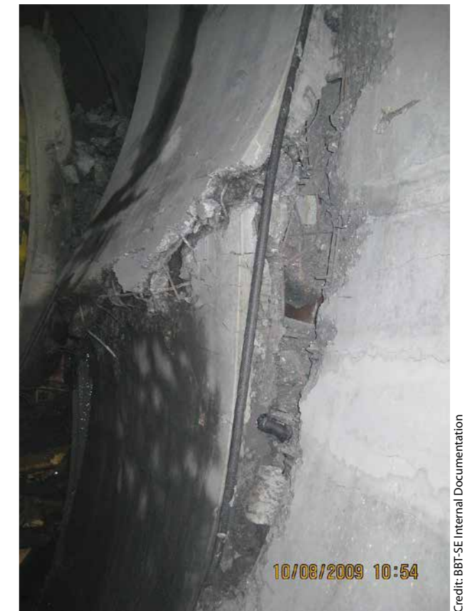
12 Aica–Mules exploratory tunnel: rupture of the segmented lining due to asymmetrical loads
