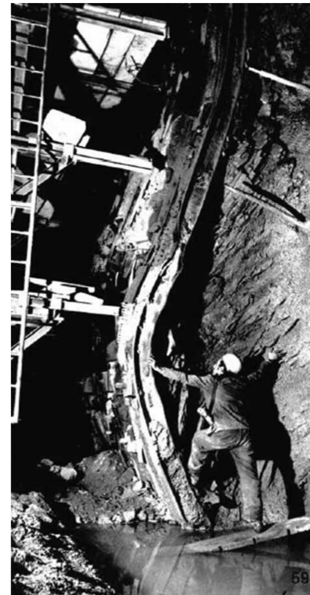
5 Druckhaftes Gebirge beim Bau des Gotthard-Strassentunnels Squeezing rock during construction of the Gotthard Road Tunnel
