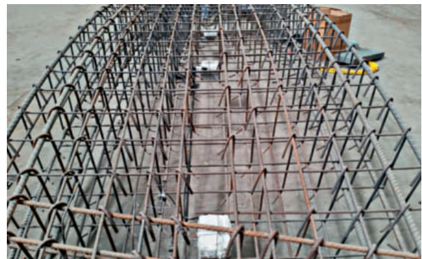
15 Installation phase of the instrument to the precasting plan for the second tunnel
