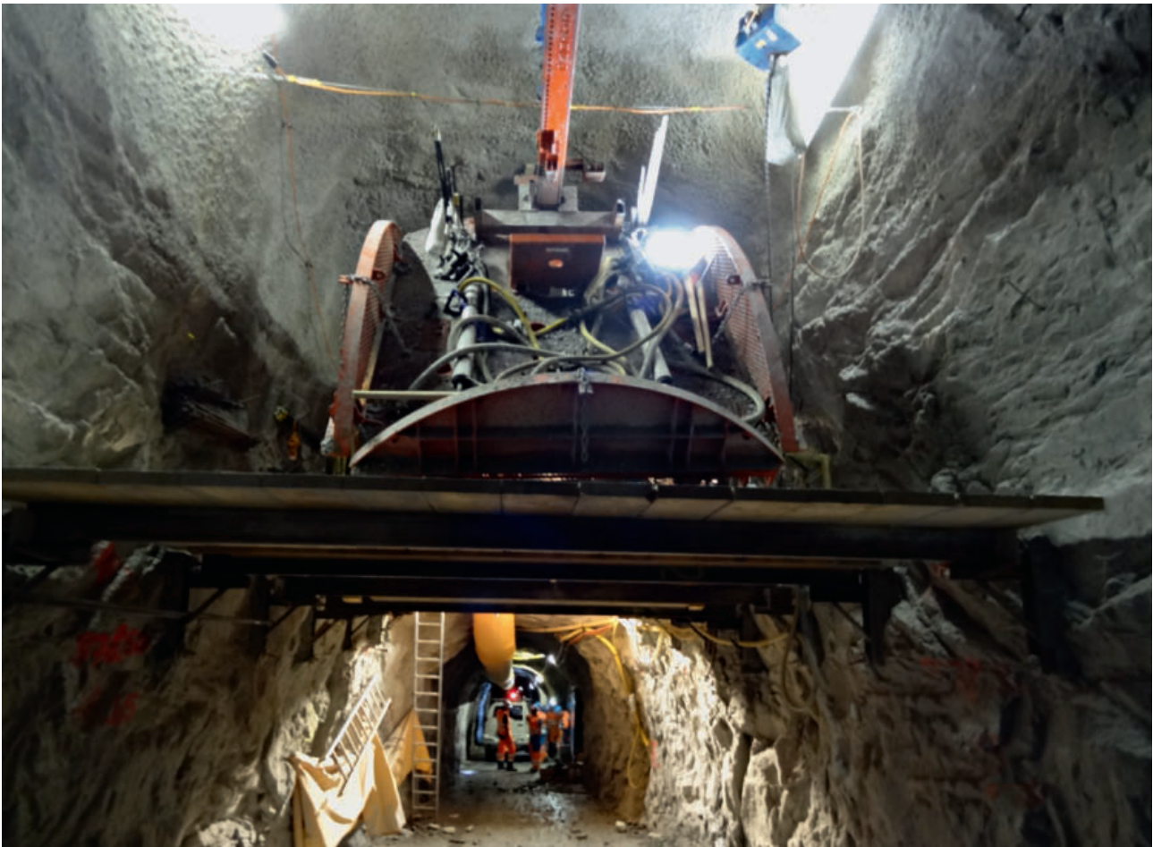
3 Alimak-Schienenkletterbühne im «Bahnhof» am Schachtfuss Handeck Alimak raise climbing platform in the 'station' at the bottom of the shaft in Handeck
