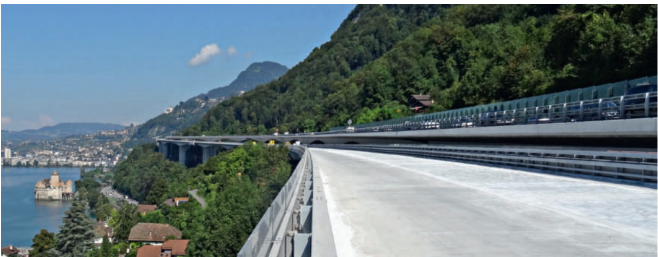
6 Fertige Fahrbahn des Chillon Autobahnviadukts zwischen Montreux und Villeneuve VD Finished deck of the Chillon highway viaduct between Montreux and Villeneuve VD
