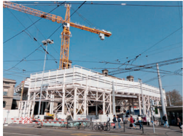
3 Installationen Südtrakt Installations at South Wing
