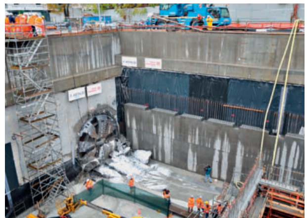
8 11.11.2014: arrivo TBM binario dispari a Forlanini FS 11.11.2014: arrival of TBM, odd track at Forlanini FS
