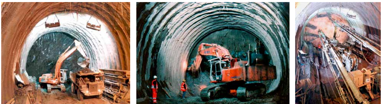
2 View of the installation of the face reinforcements and excavation phases of one of the high speed railway tunnels between Bologna and Florence (Photos: Eng. Pigorini)
