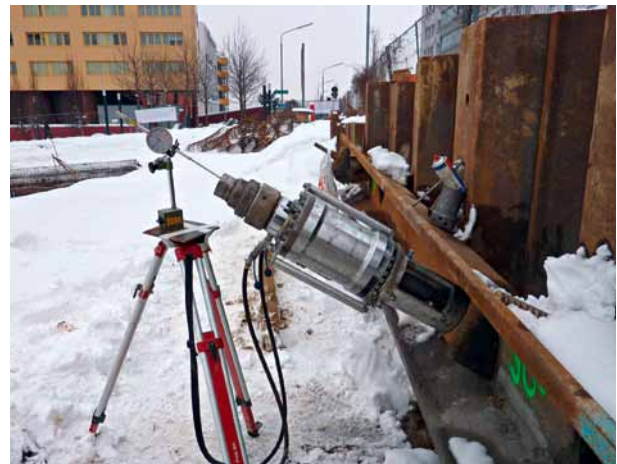
12 Example of the anchor installation during tensioning by an hydraulic jack and strain measurement (Source: Porr Bau GmbH)
