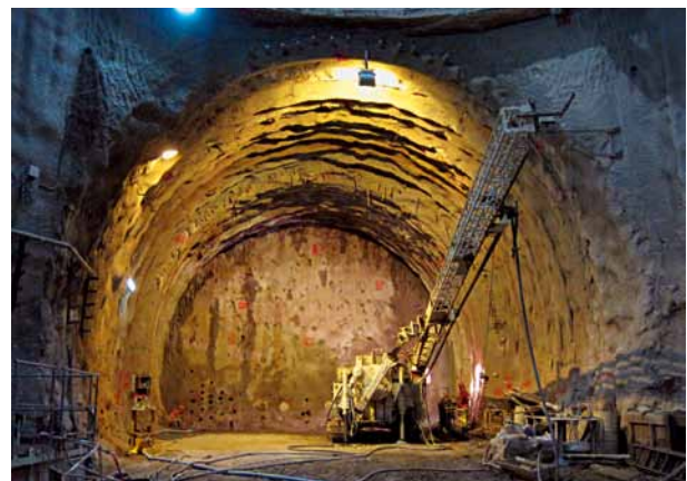
15 Tunnel face with drilling machine during the first excavation and installation of GFRP flat-bars anchors. A portion of the vertical shaft border is visible in the upper part (Source: Consolidations Suisse)
