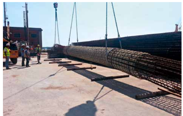
9 Napoli Port – GFRP pile cage during lifting operations (Source: Società Italiana per Condotte d'Acqua S.p.A.)
