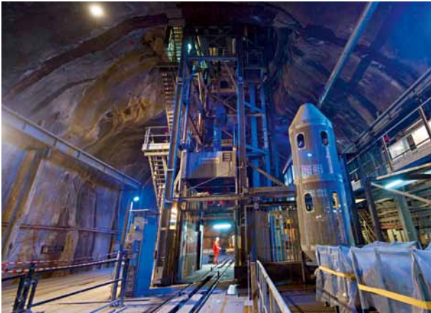
9 Beschickungsanlage Schacht 1 am Schachtkopf Charging system for Shaft 1 at the shaft head
