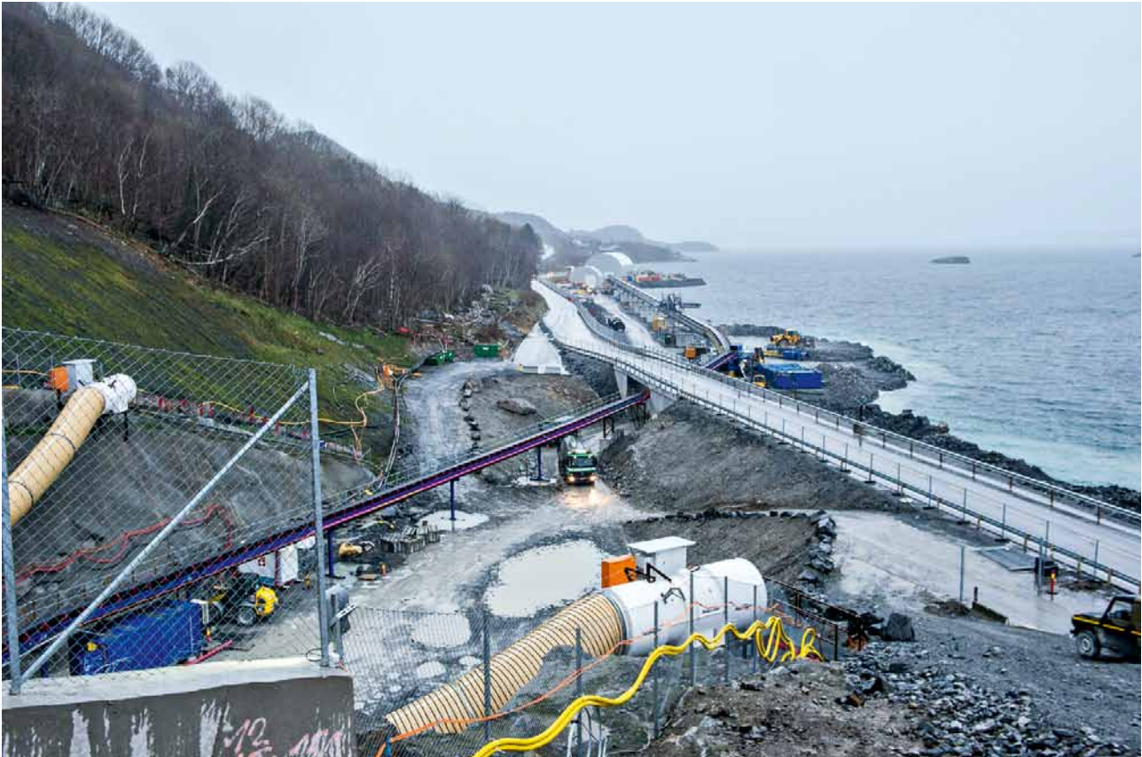
8 Bandanlage Portal Portal belt system
