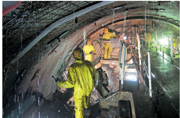
4 Erhöhter Wasserandrang im TBM-Vortrieb Increased amount of ingressing water during TBM drive
