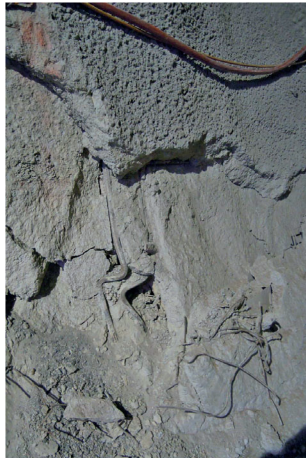
13 Fissured lining in the North-West tunnel and steel rib deformation (Tm 0-40)
