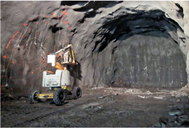
18 Front d'un intertube en cours de chargement View on a cross section during charging
