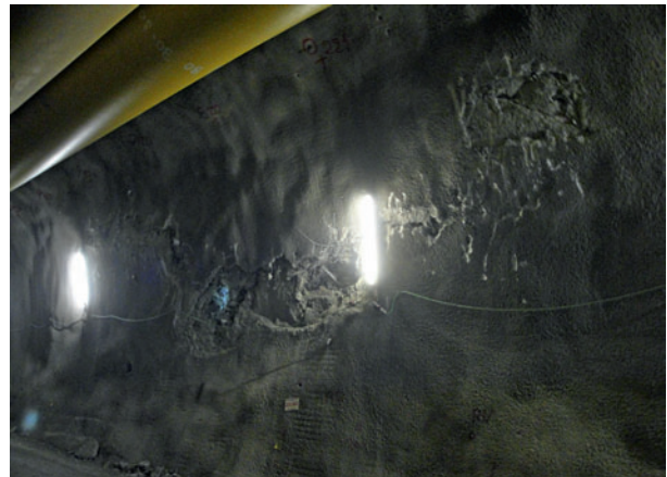
12 Fissured lining along North-East tunnel at Tm 800
