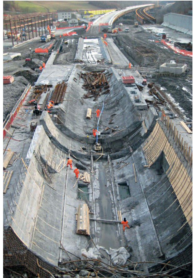
8b Facilities for housing the EPB TBM at the portal on the Florence side
