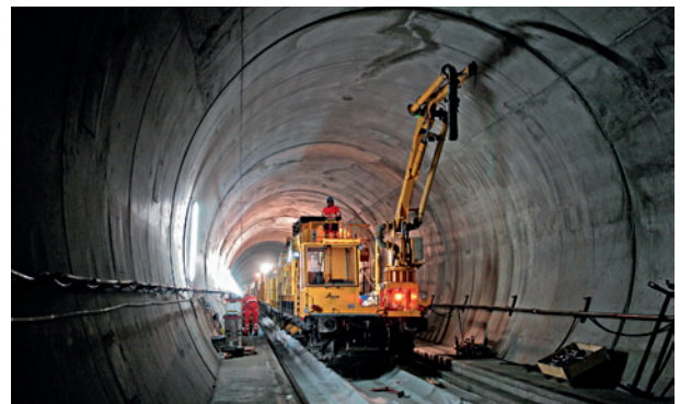
9 Pumpwagen am Kopfende des Betonzuges im Tunnel Pump wagon at the head end of the concrete train in the tunnel (Foto/Photo: TTG)
