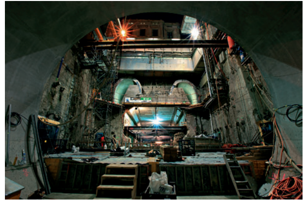
11 Blick vom Doppelspurtunnel zur „Bergmännischen Deckelbauweise“ View from the twin-track tunnel showing the “top-down construction method by mining means”
