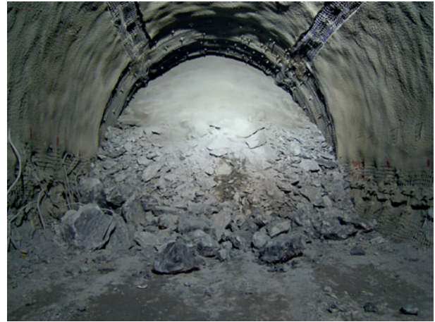
15 Full face failure occurred in the South-East tunnel at Tm 1095
