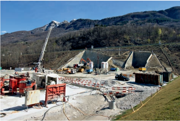
3 Bereich des Nordportals des Ceneri-Basistunnels in Camorino, Kernstück des Jahrhundertbauwerks NEAT Around the north portal of the Ceneri Base Tunnel at Camorino, the centrepiece of the NRLA project of the century Quelle/Source: ATG
