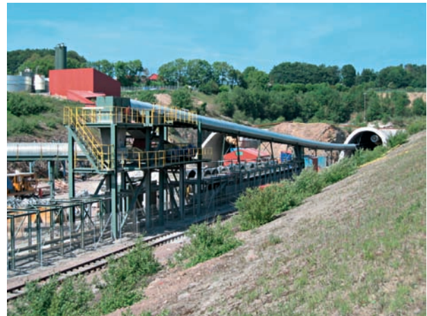
2 Tunnelbandanlage Hallandsås (S) mit Bandspeicher The Hallandsås (S) tunnel-belt installation, showing belt take-up and storage unit
