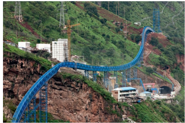
10 Kurvenband Jinping (CN) The curved belt at Jinping (CN)
