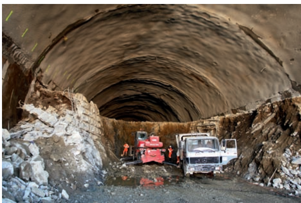
10 Portal Vigana: Strossabbau in der Kaverne Ost The Vigana portal; excavation of the bench in the East Cavern
