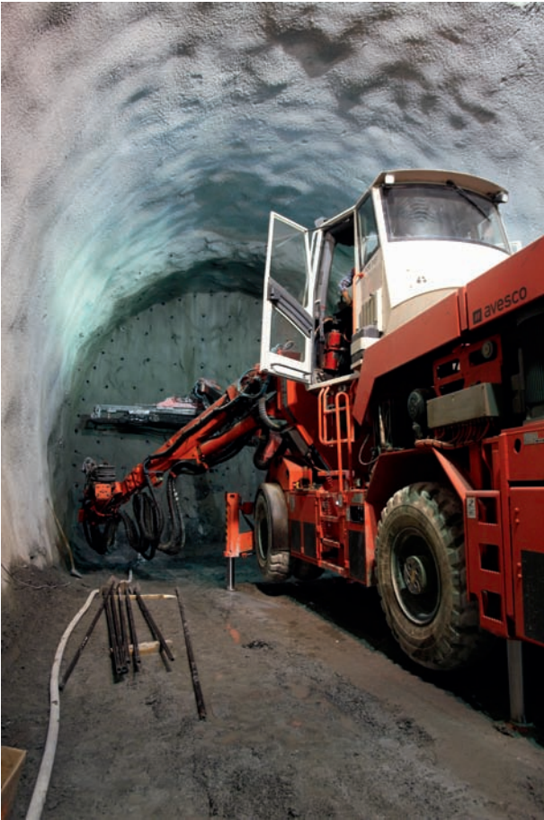
11 Ankern in der Weströhre Nord Sigrino Rock-bolting in the northern west bore, near Sigrino
