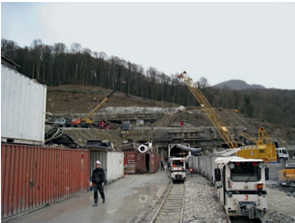
4 Nordportalbereich Eisenbahn- und Servicetunnel inklusive Risikobeurteilung The north portal zone of the rail and service tunnels, including risk assessment
