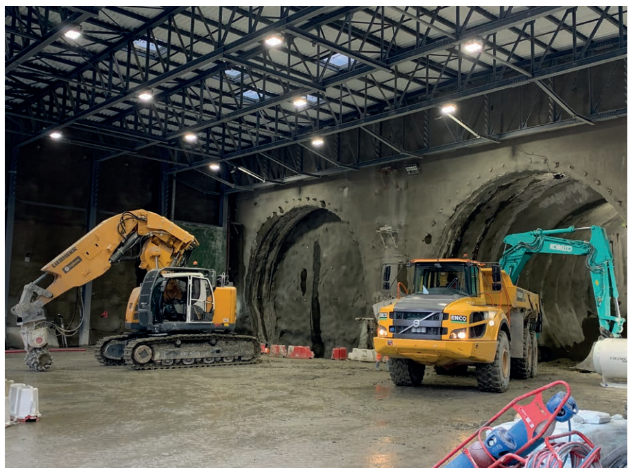
21 Start of tunnelling in December 2022 in the injected subsoil under the protection of the acoustic hangars
